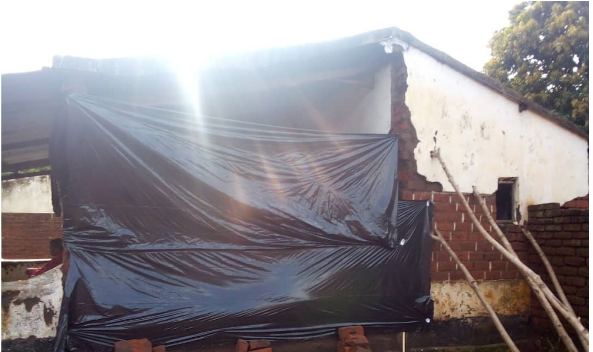
Precious Makono's house ( ST Courier for Phalombe) after being hit by Cyclone Freddy- Phalombe district (Photo taken by Precious Makono)
